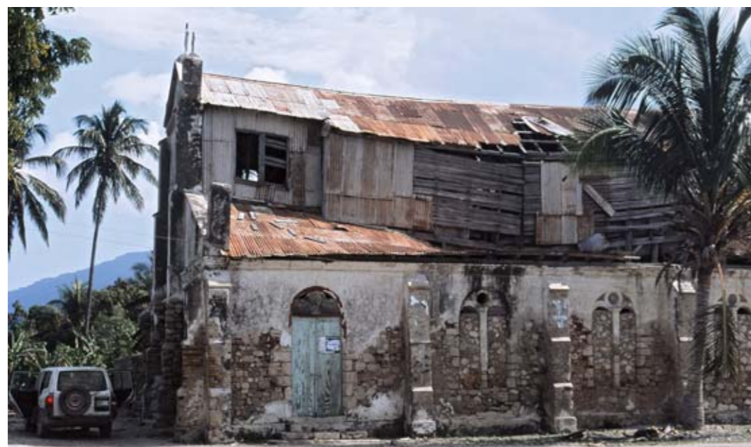
The abandoned church in Mole-Saint-Nicolas looks pathetic. There is, however, another, a more modern and functional one nearby.
