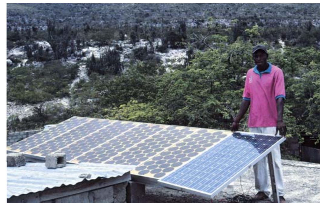
Other solar panels are installed on the presbytery. They supply power for the lighting, a computer and a refrigerator. The presbytery can also use a diesel generator to produce electricity, but the fuel is expensive and needs to be imported from far away.
