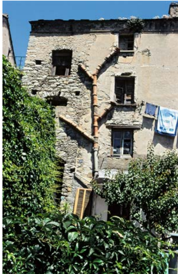
A peculiar, rather outdated sewer system.
